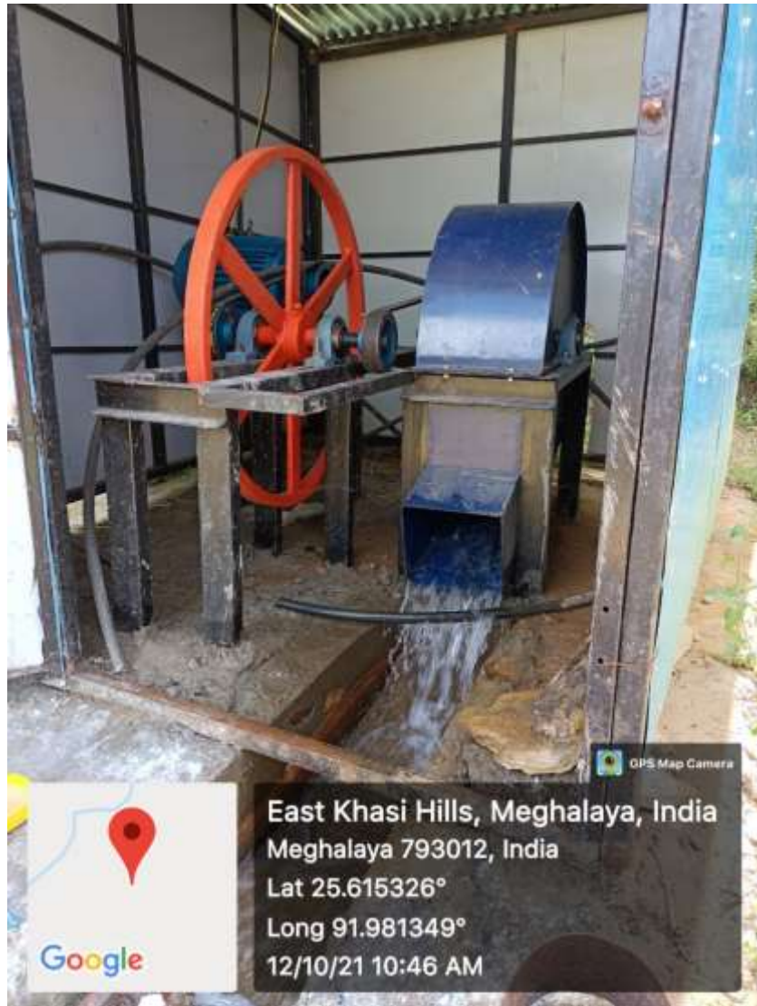
Mini-hydro power generation in Mawkasiang campus
