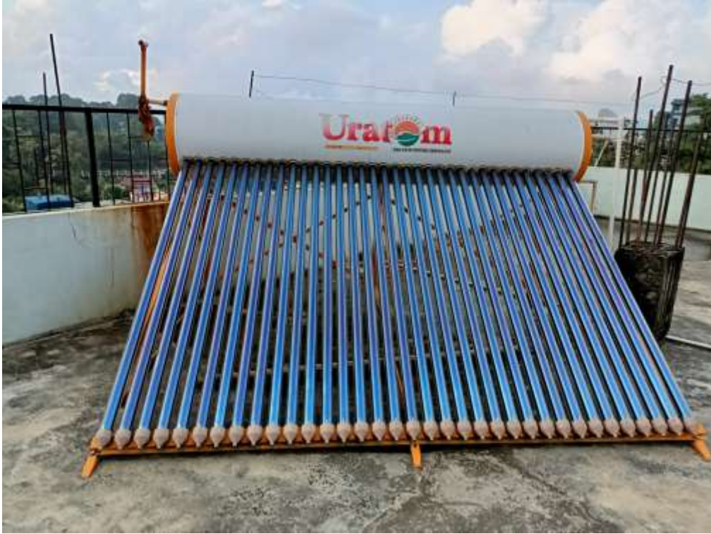
Solar water heaters in the girl's hostel
