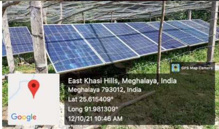
Solar power generation in Shillong College Main campus and Mawkasiang campus
